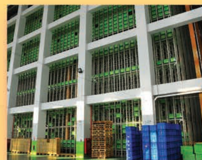
▼自動倉庫 Computer Warehousing
